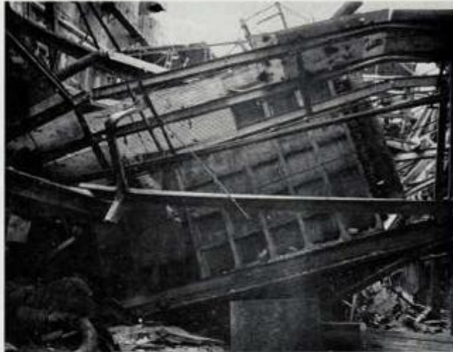
Photo 62. Building 13A. This photo was taken from the ground floor and shows the converters that have been overturned by the blast effect from the 4,000-lb. bomb described in the preceding caption.
