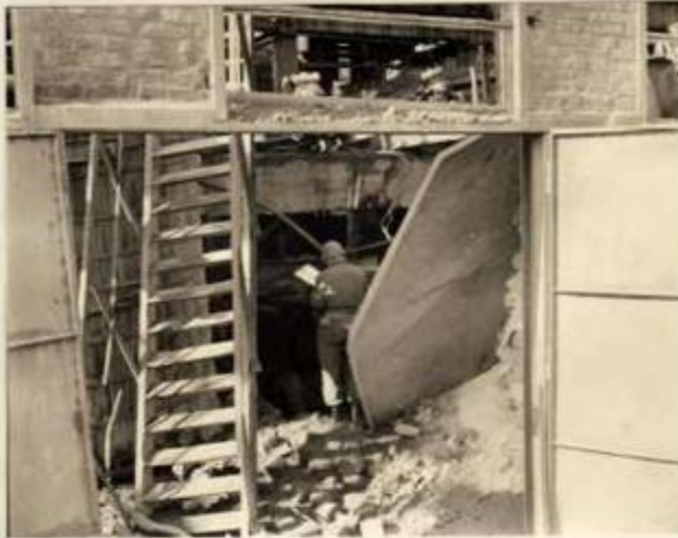
Photo No. 3. CATALYST PLANT. (Plot Plan No. 301) Bomb detonated in Bay 6. This bomb penetrated the roof in the center of the building detonating in the floor making a crater 20'x25' and 10' deep. Note fracture in the reinforced concrete girder in the first deck.
