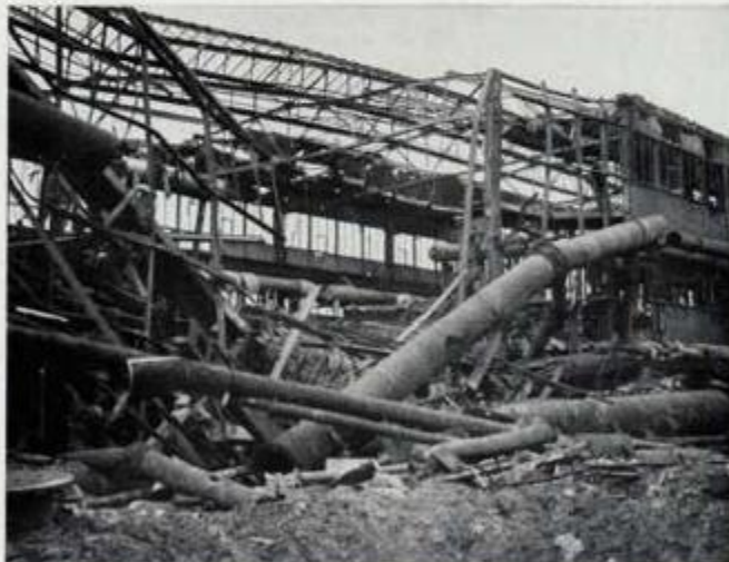
Photo 63. Building 13B. Another 4,000-lb. HE bomb detonated in the roof section of the Fischer-Tropsch reactor house shown above. Blast damage structurally destroyed the center of the building and the main piping loop as shown in the foreground.
