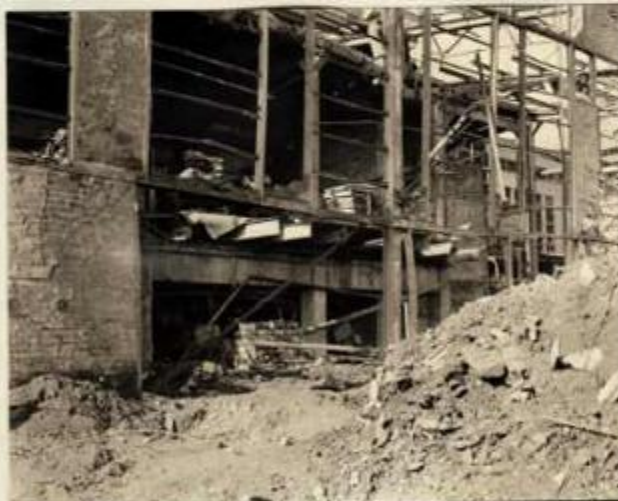
Photo No. 4. CATALYST PLANT. (Plot Plan No. 301) Bomb detonated in the ground between the equipment structure and the outside north wall. Note damage to deck plate on first operating deck and spalling of the concrete on reinforced concrete column. The damage may be considered superficial in that the structure and equipment was not seriously damaged.
