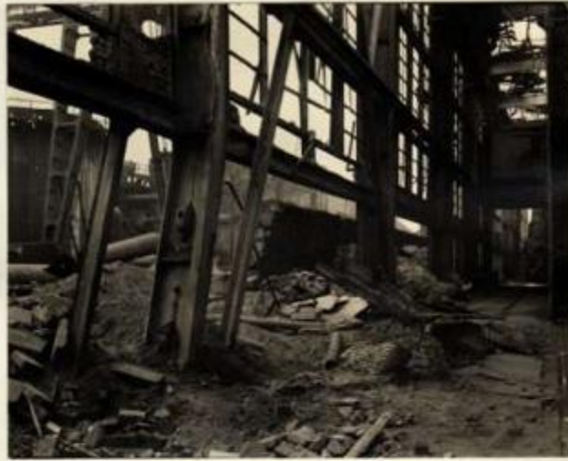
Photo No. 67. F-T CONTACT OVEN HOUSE. (Plot Plan No. 641) (Middle pressure) Blasted footing out of plumb several feet.
