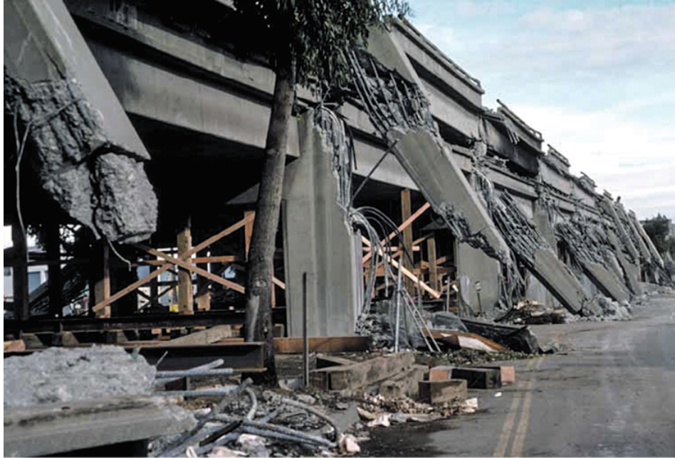
Figure 17. Cypress Viaduct in Oakland, California, after the 1989 M6.9 Loma Prieta earthquake. Source: USGS
